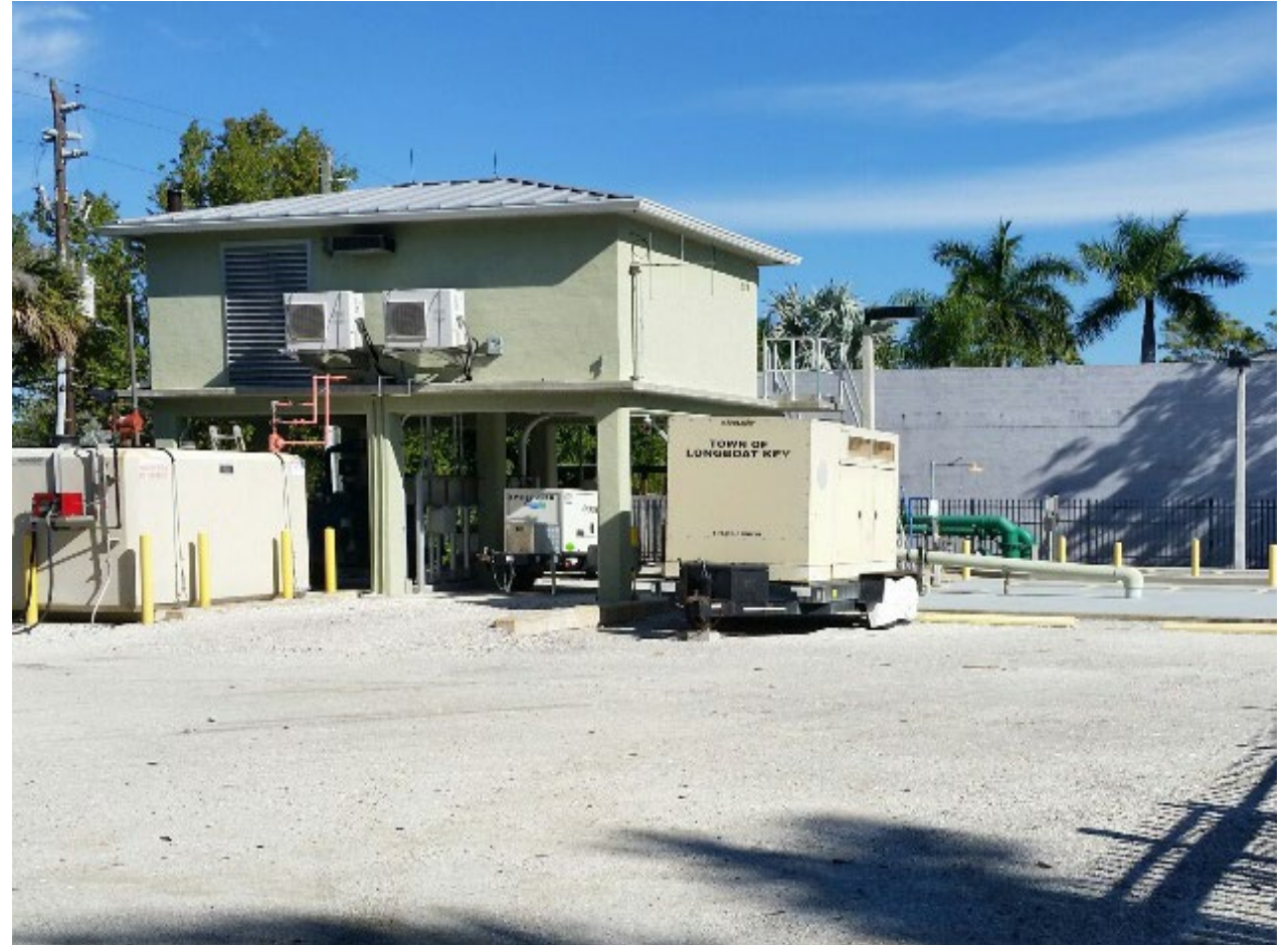
Master Lift Station D – Gulf Bay Road
