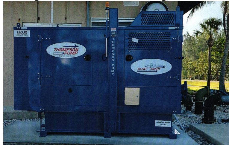
Lift Station "E" By-Pass Pump
