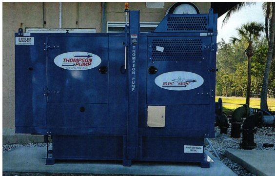
Lift Station “E” By-Pass Pump
