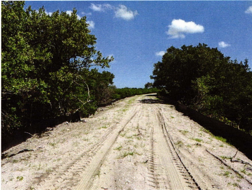
Photo #7 – Temporary repair haul road looking North (towards intertidal and freshwater interface).
