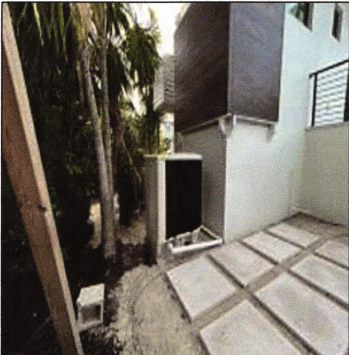
AIR CONDITIONER PHOTO TAKEN ON JANUARY 22, 2024
