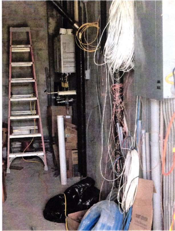
Tank Less Hot Water Heater
