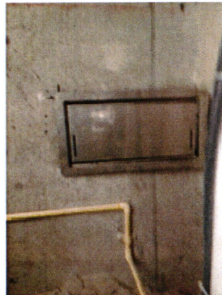
SMART VENT UNDER A/C PAD (1):
