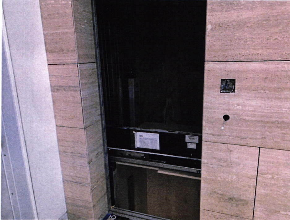
(3/13/2021) Elevator Equipment Located on Top of Elevator
