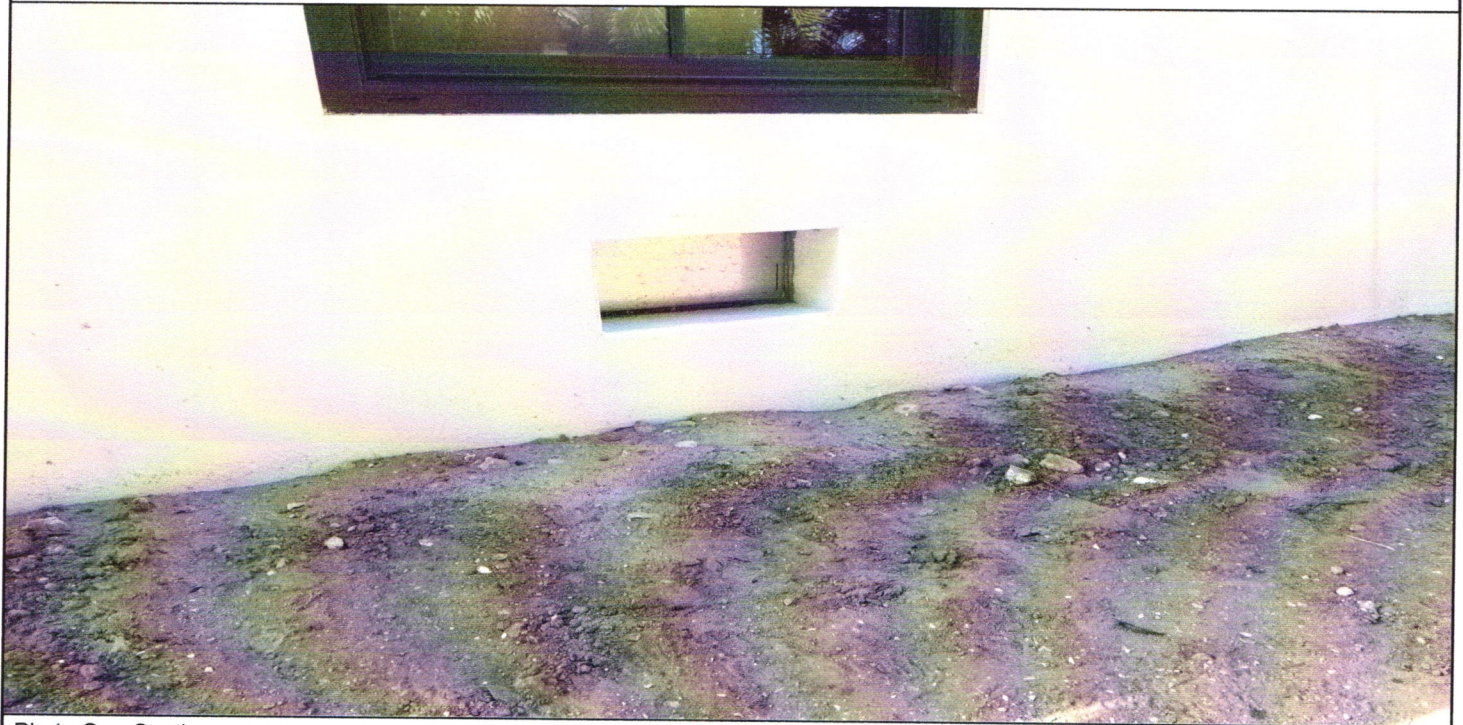
Photo One Caption 585 Channel Lane - Vent Photo
