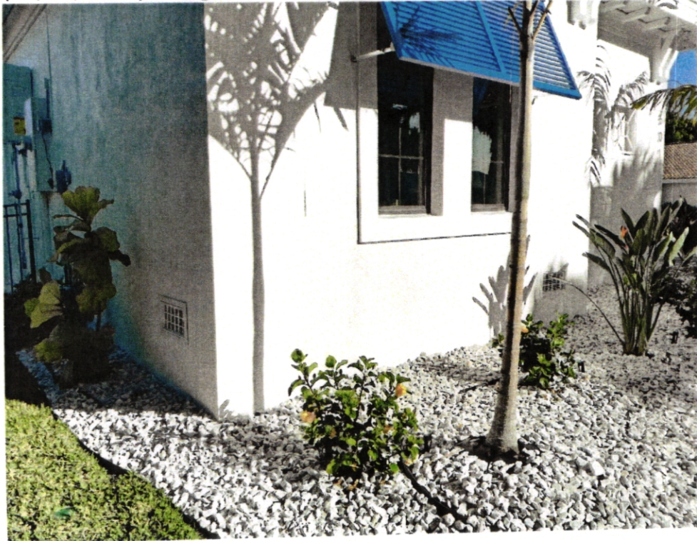
(04/25/2024) 1 Engineered Flood Flap Vent Front in Garage Wall
