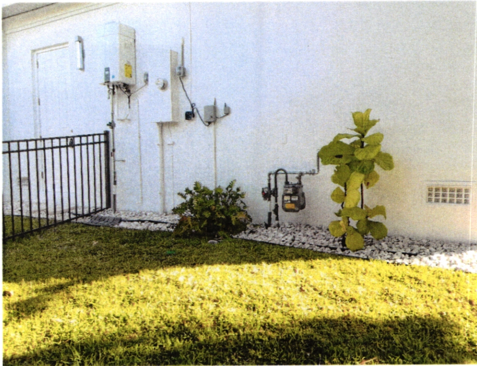
(04/25/2024) 2 Engineered Flood Flap Vents Left Side in Garage Wall, Tankless Water Heater on Wall =13.1'
