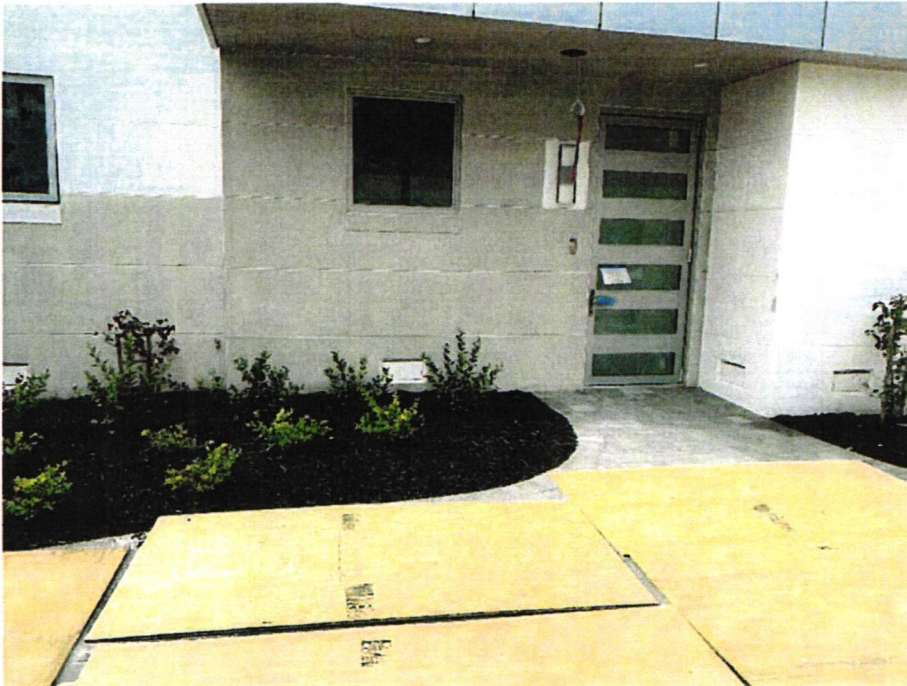
(01/03/2024) 4 Smart Vents Model #1540-520 in Front View of Entry/Elevator Area
