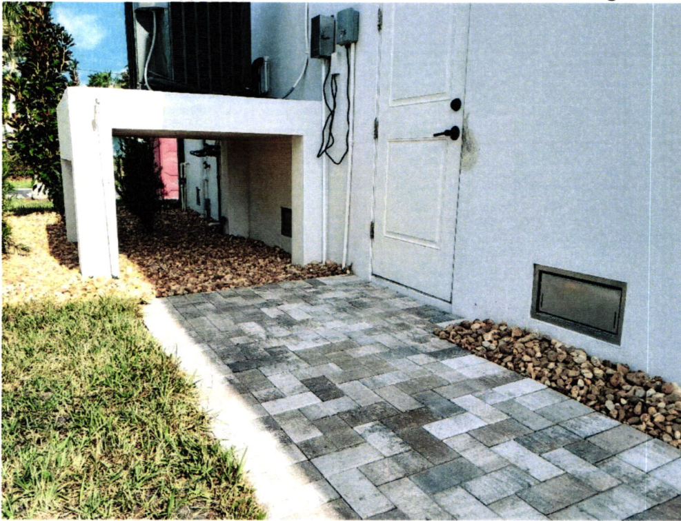
(11/21/2023) 3 Typical Smart Vent Model #1540-520 on Right Side Wall of Garage
