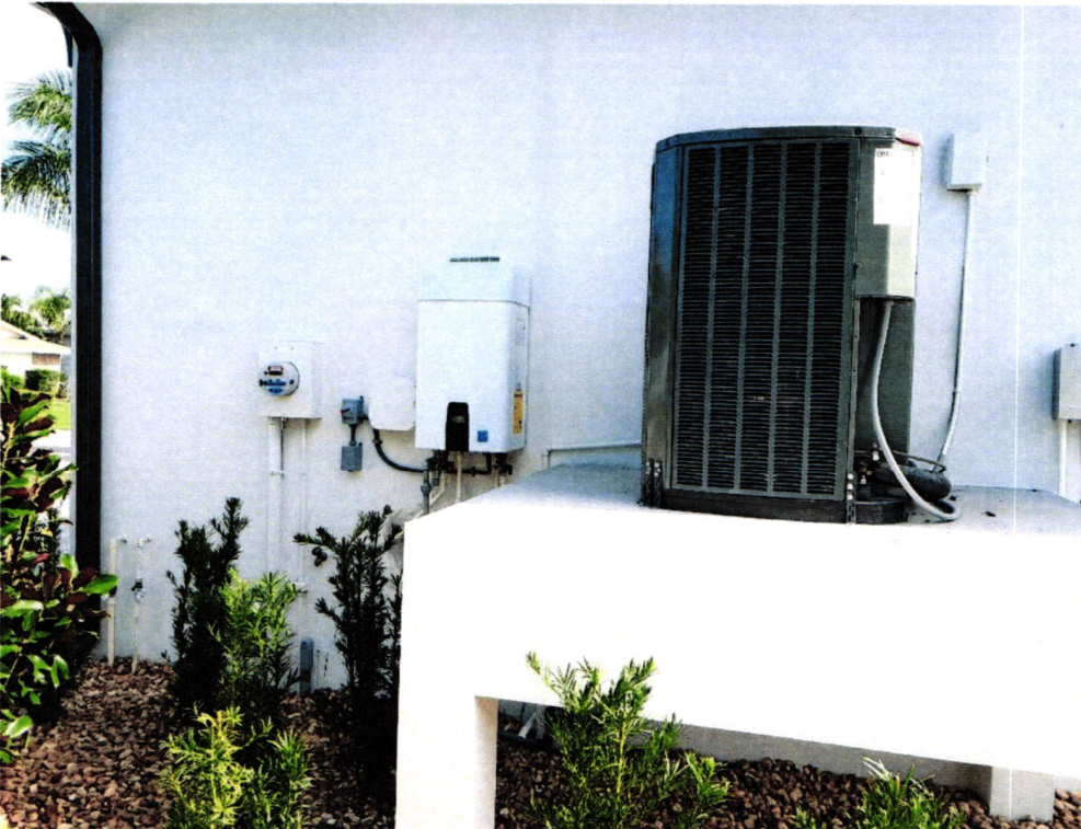
(11/21/2023) Elevated AC Platform= 9.0', Tankless Water Heater= 9.3'
