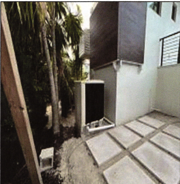
AIR CONDITIONER PHOTO TAKEN ON JANUARY 22, 2024
