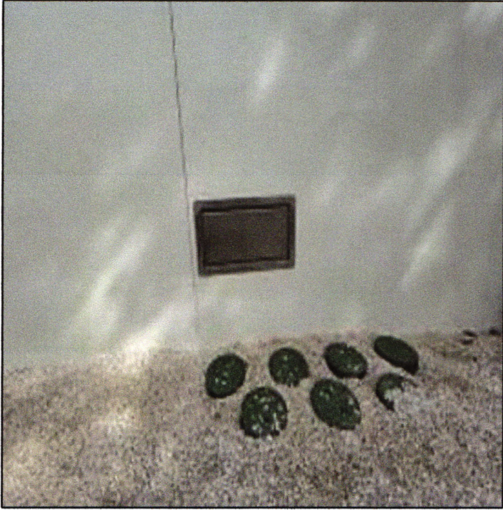
VENT PHOTO TAKEN ON JANUARY 22, 2024
