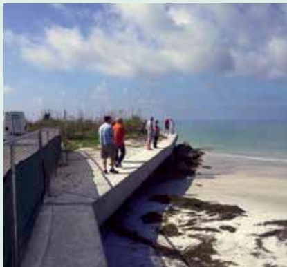
The panel inspects a washed-out beach off North Shore Road.
